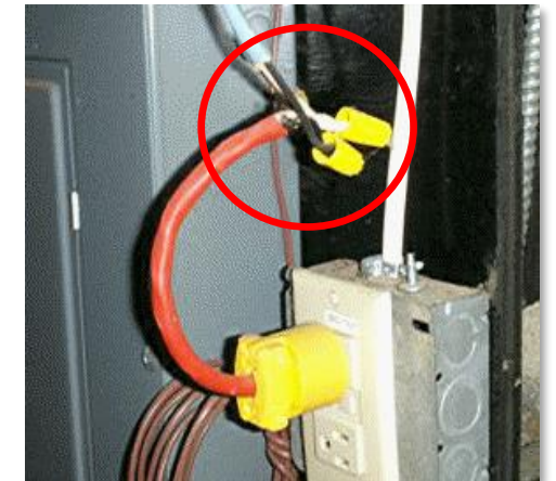
Spliced electrical cords
