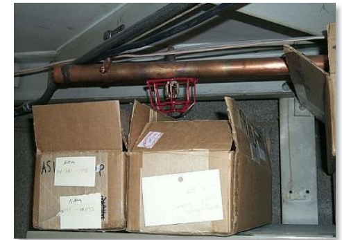
Blocked sprinkler heads
